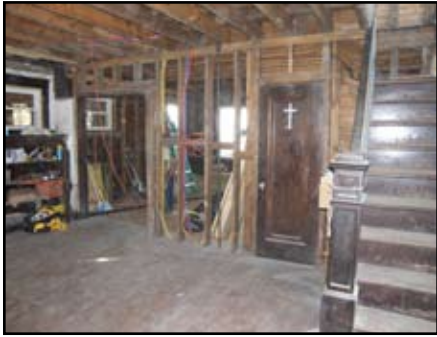
Ministry volunteers installed drywall, scraped, and painted in April and May at the Fairmount Ave. house.
